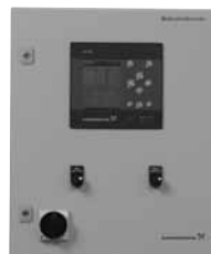
Fig. 3 Grundfos Dedicated Controls
